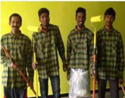
Burmese Asylum Seekers painting the walls of the new Asylum Seeker Resource Centre in Dandenong, Victoria. Photo courtesy of ASRC
